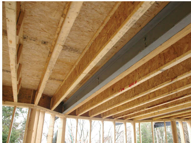
Figure 3. On this project, four MC-10-22 steel beams were bolted to the interior joists on 8-foot centers.
