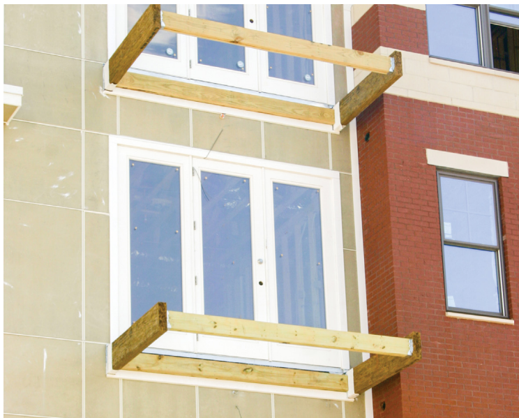
Figure 7. Instead of a system of cantilevered joists connected to the interior floor framing, these balconies are framed with pairs of cantilevered LVL beams.
