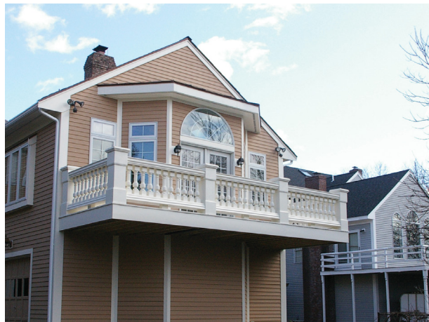
Figure 5. Unlike a deck's 36-inch minimum railing height, a balcony's railing is required by code to be a minimum of 42 inches high.
