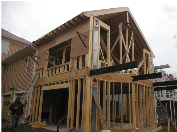
Figure 2. Structural steel can be used to frame wider balconies, though steel often requires specialized or unfamiliar techniques and can be more expensive than wood framing.
