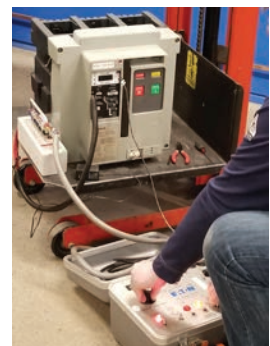
Secondary Injection Testing
