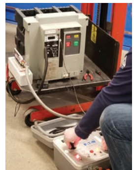
Secondary Injection Testing
