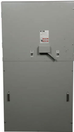
Main circuit breaker 3MFS1200RUG
