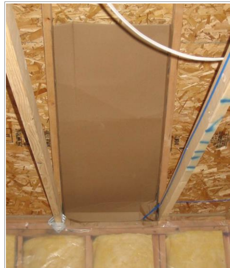
R402.2.3 Eave Baffle Baffle at eave vent. Minimum 1" unobstructed air space required.
