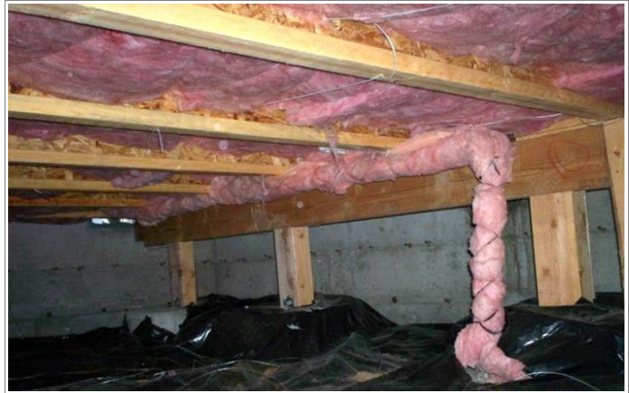
R402.2.7 Floors Floor insulation installed with contact to the underside of the floor decking. Note the inset stapled twine.
