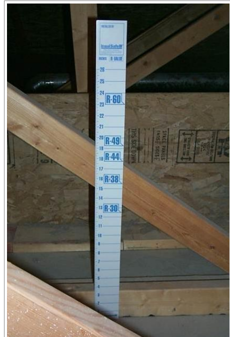
R303.1.3 Insulation Markers Insulation marker installed in attic. Make sure the marker is applicable to the type of insulation installed (fiberglass, cellulose, etc.).
