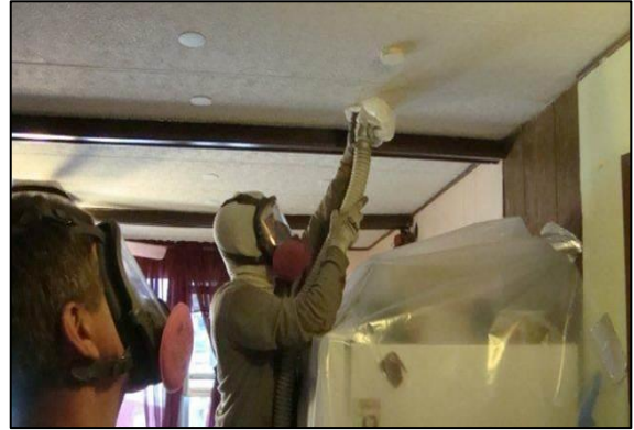
Installing insulation through the ceiling: The technician pushes the fill-tube into the cavity and out near the edge of the roof. The holes are drilled in a straight line for appearance sake.
