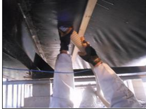
Blowing insulation from under the home: A large diameter fill tube fills cavities rapidly from underneath.
