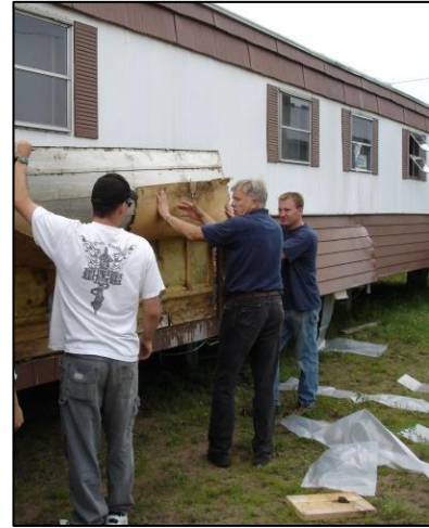
Loosening siding for wall insulation: Remove screws at the bottom of the metal siding. Before installing insulation, fasten the siding sheets together at the bottom with a short sheet-metal screw.
