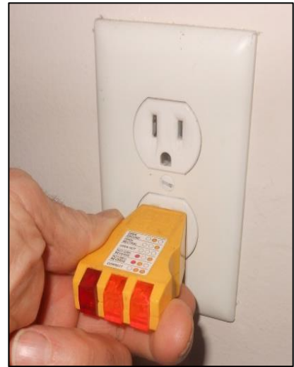
Checking walls: Measure the cavity and the existing insulation level. Make sure wall outlets work before and after insulation installation.
