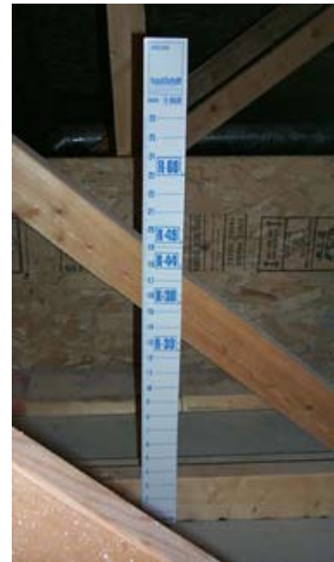
Figure G-1 Insulation depth marker
