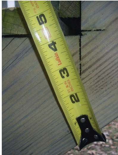
Figure 5. A 2x12 stringer has a maximum unsupported span of 6 feet. These stairs are likely to deflect and cause the stringers to either pull loose from the framing or shear along the grain (far left). The problem is made worse with overcut notches, which weaken a stringer. The minimum recommended depth of the uncut portion of the stringer is 5 inches, as measured to the closest saw kerf, and not the notch itself.
