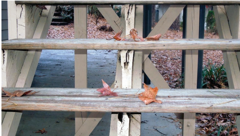
Figure 6. Stairs that are higher than 30 inches off the ground are subject to the same guidelines as railings, so avoid open risers that permit the passage of a 4-inch-diameter sphere.
