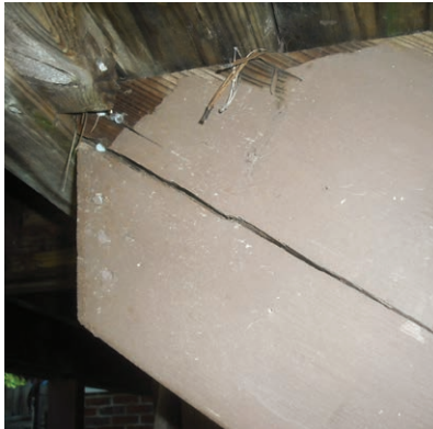
Figure 3. Stringers require adequate bearing on either a rim joist or a dropped header. Without it, the risk is that the stringer will split along the grain (left). The photo on the far left is new construction that was approved by the local building inspector.
