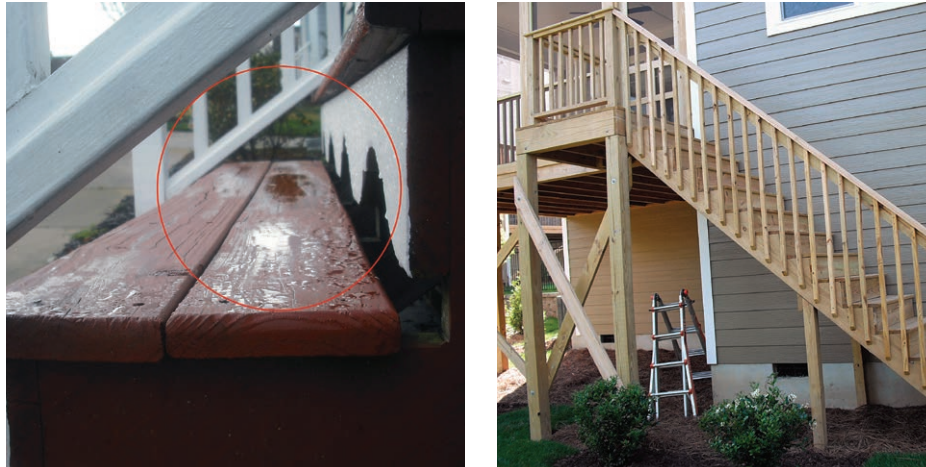
Figure 8. Bottom guard rails on stairs should be oriented close enough to the tread nosings so that a 6-inch-diameter sphere will not pass through the triangle created by the riser, tread, and rail (far left). Wooden stair guard posts should be located so that the span between posts (as measured horizontally) is no more than 6 feet. This is a new deck that passed inspection (left).
