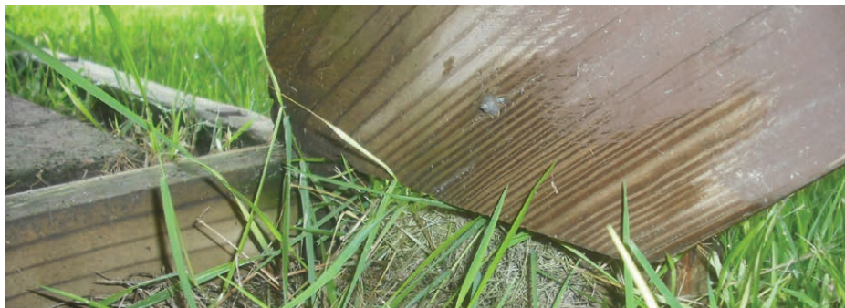
Figure 2. Allowing the toe of the seat cut to be the only part of the stringer that bears on the landing can cause the stringer to shear along the wood grain. At least 1 \frac{1}{2} inches of the heel of the seat cut should bear on the landing.
