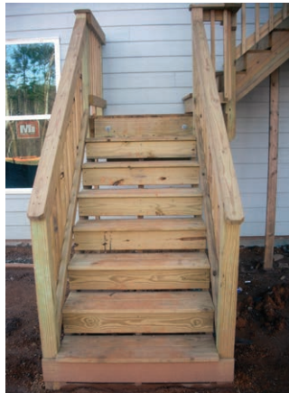
Figure 10. Avoid notched posts, which may develop cracks originating in the corner of the notch and running parallel to the grain, which weakens the post (far left).
