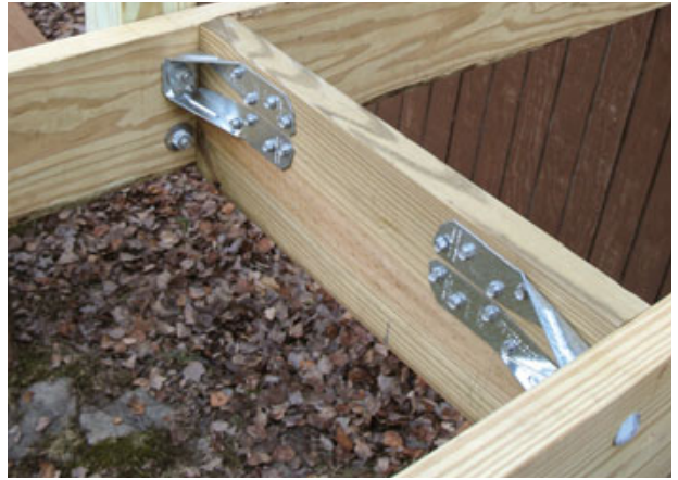
Figure 1. Once a standard engineering safety factor is applied, specialized hardware may be the only practical way to mount guardrail posts capable of withstanding the code-required 200-pound load.
