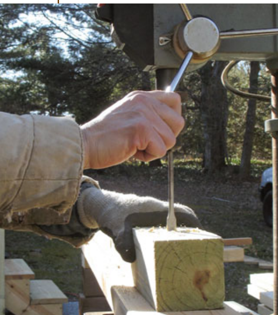
Figure 5. A small drill press set up with a plank to support the posts makes for fast, accurate, and nearly effortless boring.
