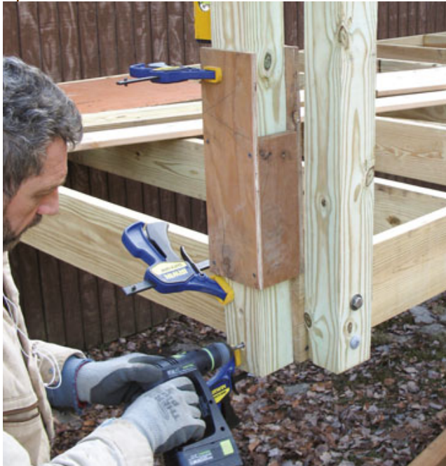
Figure 7. A box made from scraps clamped to the post acts as a positive stop to hold the post at the right height. Additional clamps secure the post to the rim, whose bolt holes are then drilled using the holes in the post as guides.
