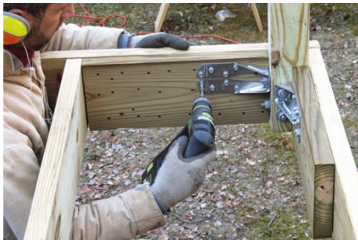
Figure 3. Most manufactured railing systems require posts mounted inside the rim. That requires both a bracket to resist the outward force at the top of the rim, and blocking to resist the inward force at the bottom of the post.
